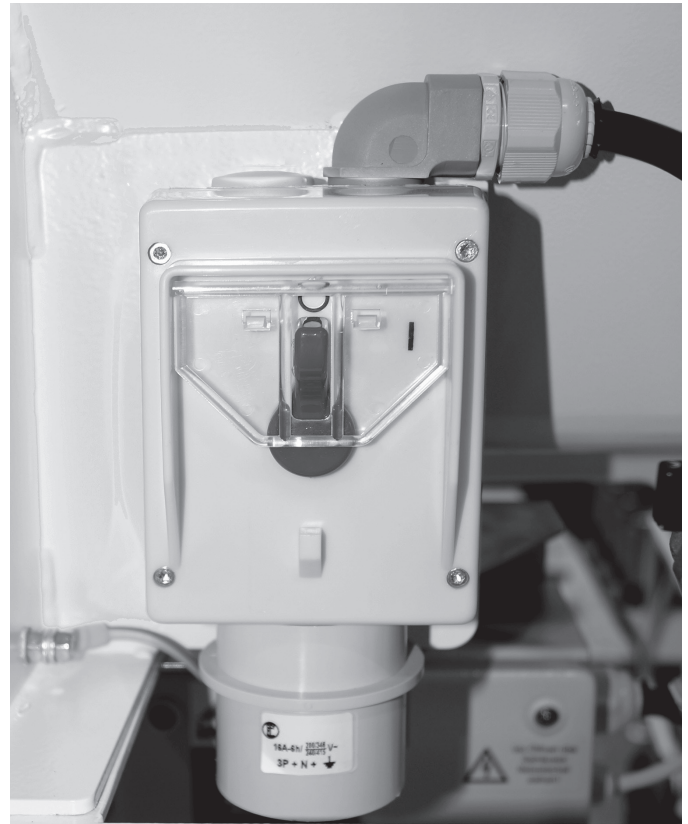
Power connection at the main switch (400 V / 16 A)
